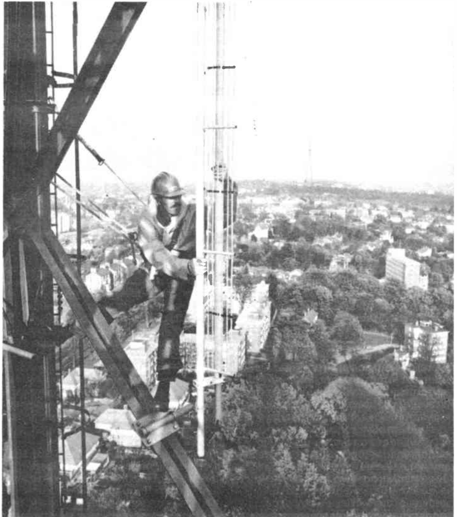
Rick Boran, an engineer from British Telecom's Mobile Communications division, fits a Cellnet antenna on the IBA transmitter tower at Beulah Hill, south London
