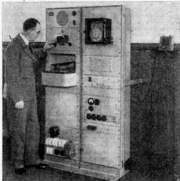
Main Equipment Rack at the Institution for the Blind. The radio receiver and record player are immediately below the loudspeaker grille, with the "programme" timeswitch at top of the right-hand rack. A microphone for local announcements can be seen on the wall.
