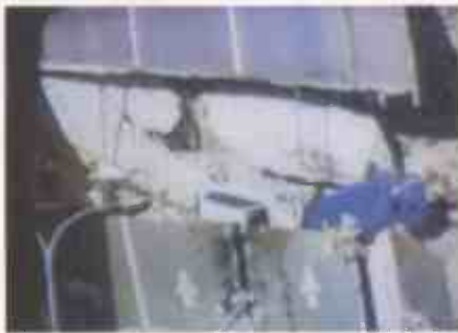
Motorway bridge collapse across carriageway crushing cars (W1)
