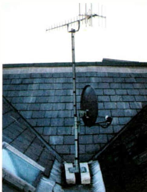
Figure 16: A groundstand with a small base and no diagonal supports has very little strength. It should be used to support only a very modest load, and even then it needs to be bolted to a large piece of concrete, not to a pair of path edgings like this. It was possible to push this installation over with one finger!
