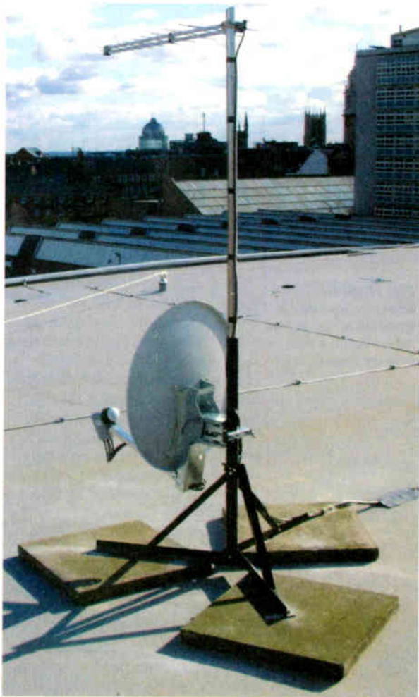
Figure 15: This 65cm dish and log-periodic UHF aerial are fixed on to a steel groundstand. The groundstand is bolted to three concrete slabs which stand on rubber sheeting to protect the roof membrane.
