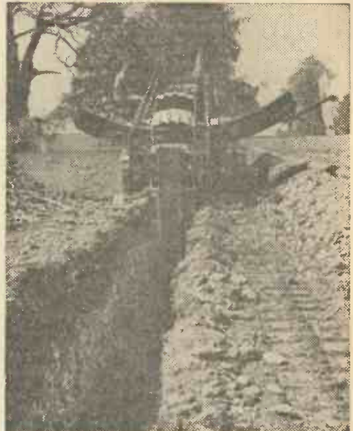
A trenching machine at work near Box in Wiltshire. Normally the line is laid at a depth of 3½ to 4ft, although this may vary slightly with differing soil conditions.
