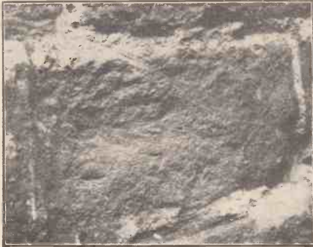
An isolated brick which has been reduced to a powdery condition by salt absorption from a badly drained subsoil.
