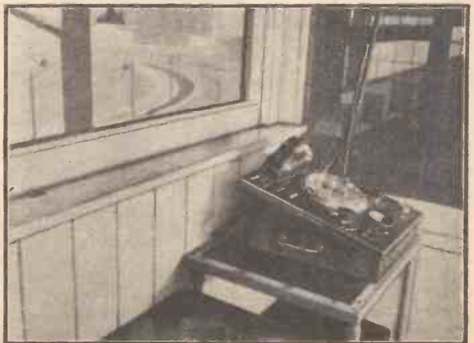
The photo-electric equipment installed in the Judges' Box at Hackney Wick Stadium, London.
