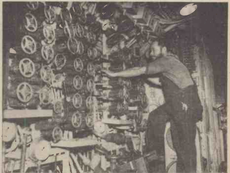
An engineer operating some of the controls on one of H.M. submarines. Note the multiplicity of valves and dials.
