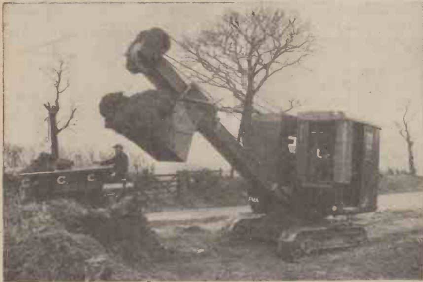
Fig. 4.—A ½ yd. skimmer on road widening work. (By courtesy of T. Smith and Sons, Ltd.)
