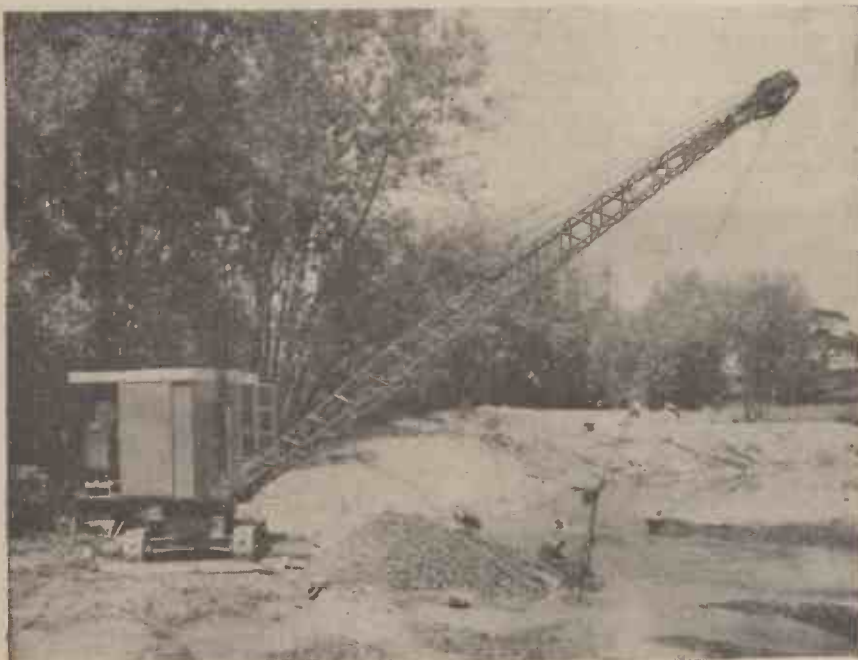
Fig. 5.—A 17ft. dragline on river widening work. (By courtesy of T. Smith and Sons, Ltd.)
