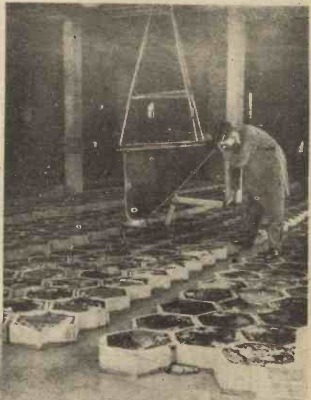
Asphalt mastic being run out from a mechanical mixer and cast in steel moulds.
