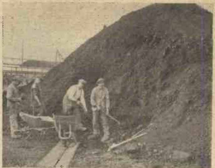
The commencement of manufacture. Native Cuban asphalt being collected from a stock pile for processing.
