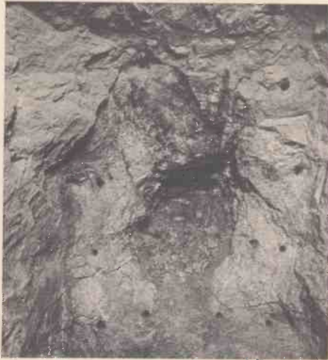
A rock face showing holes drilled ready for the insertion of detonators
