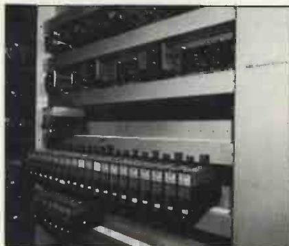
Type RR Reed (FDM) remote control equipment at Waverley signalling centre
