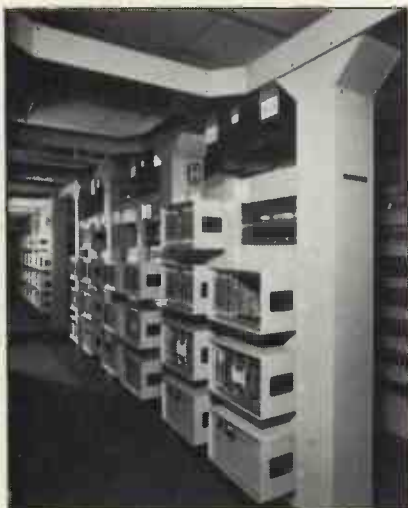
Type RM (TDM) remote control equipment at Victoria signalling centre
