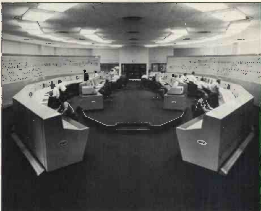
The Victoria signalling control centre and train describer for British Rail Southern Region
