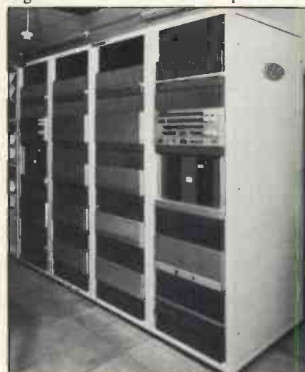
Train describer cubicles at Victoria signalling centre
