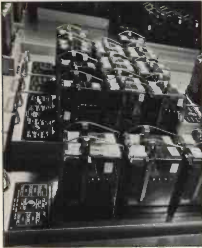
Geographical route relay interlocking at Waverley signalling centre
