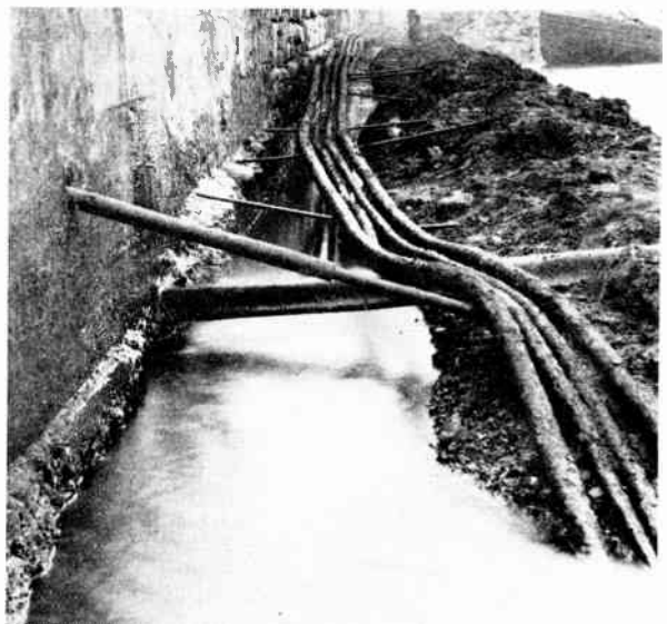
Fig. 45.—JOHNSON AND PHILLIPS' SUBMARINE CABLES REMOVED FROM WEYMOUTH HARBOUR TO NEW POSITION ABOVE HIGH WATER LEVEL AFTER 25 YEARS IN SALINE MUD.
