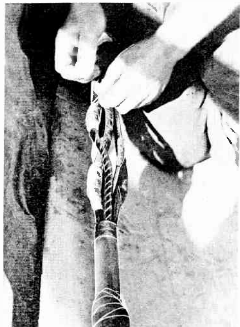
Fig. 49. —L.T. STRAIGHT-THROUGH CABLE JOINT—FOURTH STAGE. Showing lincn tape being applied to joint ferrules.
