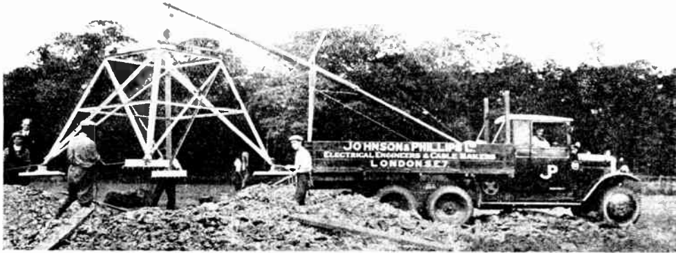
Fig. 22.—LIFTING STUBS FOR STRAIGHT LINE TOWER ON 33,000-VOLT LINE. The stubs are guided by ropes at each corner.
