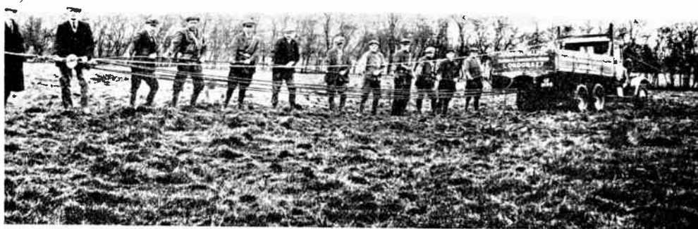
Fig. 16.—PULLING CONDUCTOR UP TO TENSION BY MEANS OF DYNAMOMETER AND ROPE BLOCKS.
