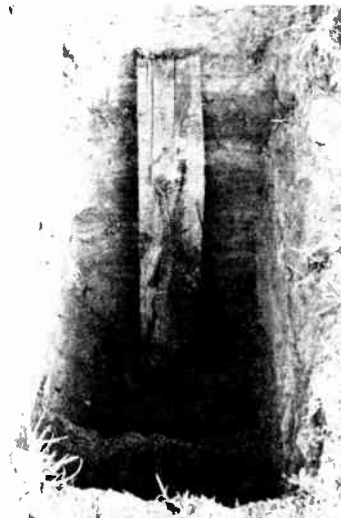
Fig. 8. — SHOWING STEPPED POLE HOLE AND SKID PLANK FOR THE POLE BUTT TO SLIDE DOWN.
