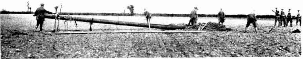
Fig. 10. —ERECTING E.H.T. POLE—FIRST STAGE. Showing pole lifted on to trestle, gin pole erected and men ready to pull up.
