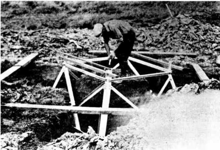
Fig. 23.—LEVELLING THE STUBS BY MEANS OF TEMPORARY LEVELLING RODS ON THE STUB ANGLES.
