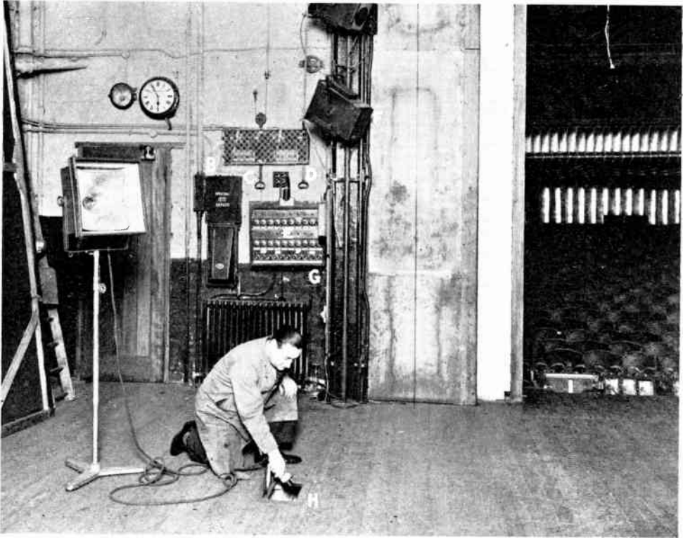
Fig. 4.—A VIEW OF THE PROMPT CORNER AND VARIOUS SECTIONS OF STAGE LIGHTING. A, wing flood; B, special effect; C, fire curtain control; D, sprinkler control; E, signal board; F, "times"; G, prompt corner; H, dip.
