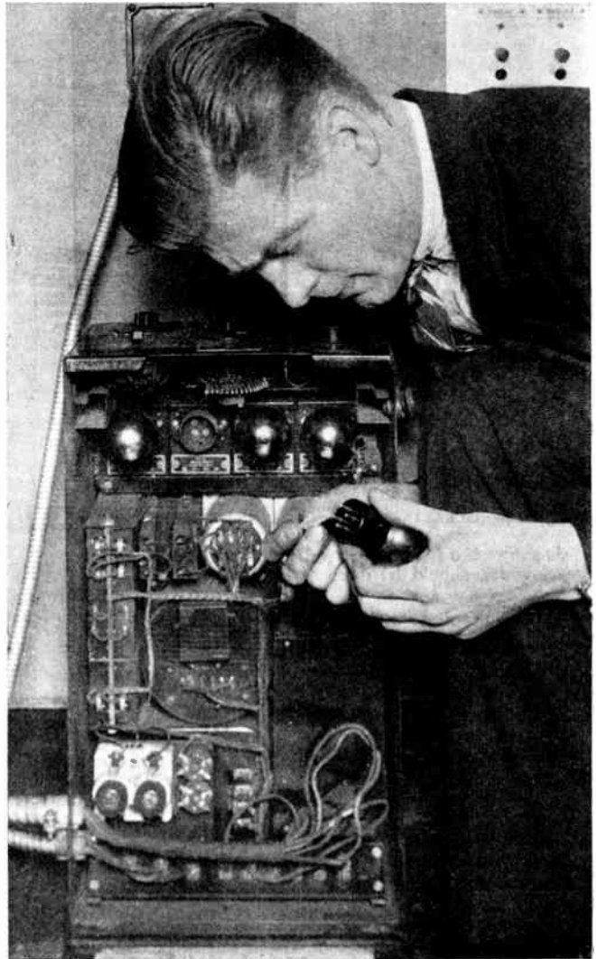
Fig. 13.—CLEANING LEGS OF VALVES OF MOTOR CONTROL BOX. This should be done once a month.
