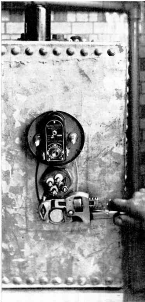
Fig. 7.—FINAL FIXING OF FLANGE, COMPLETE WITH IMMERSION HEATER AND THERMOSTAT, TO HOT WATER TANK.
