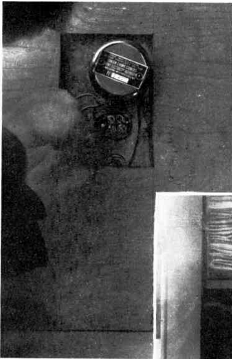
Fig. 9.—FINAL CONNECTIONS BEING MADE TO IMMERSION HEATER, SHOWING ALSO WOOD BOX ROUND TANK CONTAINING LAGGING.
