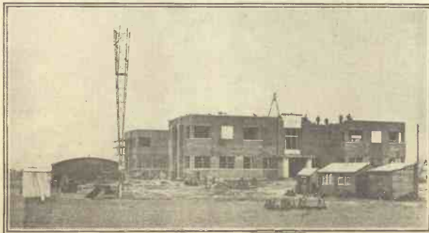
The special anti-fading aerial in course of construction at the Northern Ireland Regional station at Lisburn. The effects of this aerial will be watched with interest, and, if successful, may lead to modifications of existing aerial systems.
