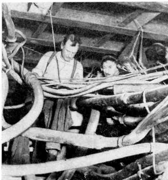
Somewhere in this maze of cables which is being moved to make room for the new Underground Railway station at Holborn, London, are the all-important B.B.C. telephone circuits! Actually 70,000 telephone circuits in 100 cables are involved, and during the alterations not a single circuit will be interfered with or put out of service.
