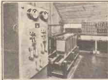
Quite a considerable space is occupied by the power plant at the Lisbon CT1AA station, the large accumulators near the middle of the picture being the 18-volt L.T. supply. The charging-board for this is in the foreground, and in the background can be seen part of the 5000-volt High-Tension equipment.
