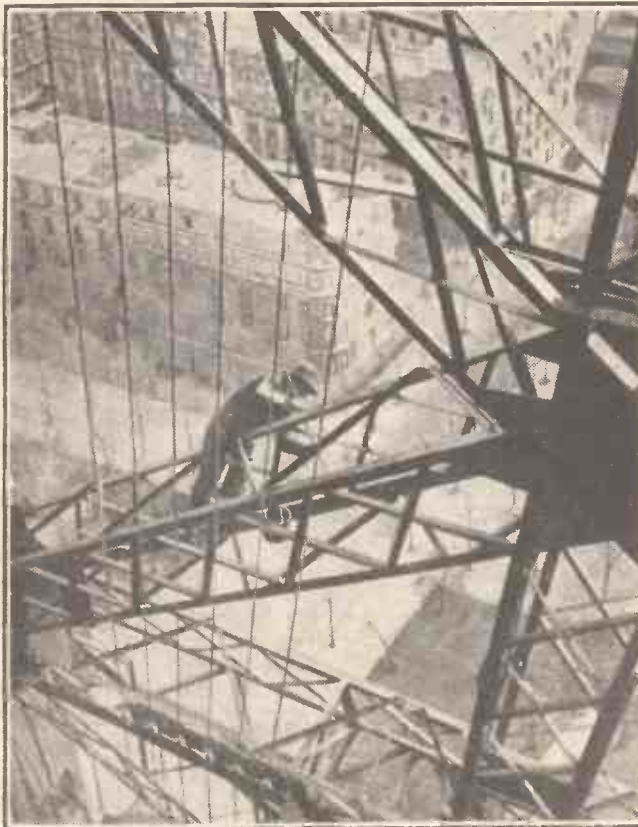
Paris has decided that the famous Eiffel Tower deserves a new coat of paint, and here is a picture of French roof tops and of one of the workmen with his paint-pot and big brush. The Eiffel Tower transmissions go out on a wave-length of 1445.7 metres.
