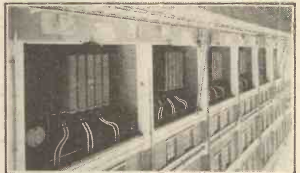
Besides making parts for your set, the Ferranti people build colossal electrical gear, such as the transformers seen above, which are installed in the Birmingham Corporation's new generating station. They handle up to 33,000 volts.
