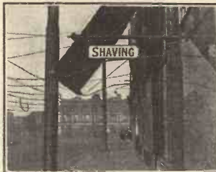
A flashing electric sign which produced much interference, but which was cured by placing fixed condensers across its contacts.
