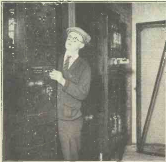
One of the engineers adjusting the radio-telephone modulation apparatus at the Rugby Station.
