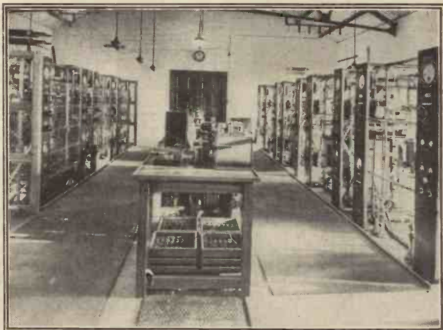
The control table in the transmitting hall of the Grimsby Beam Station.
