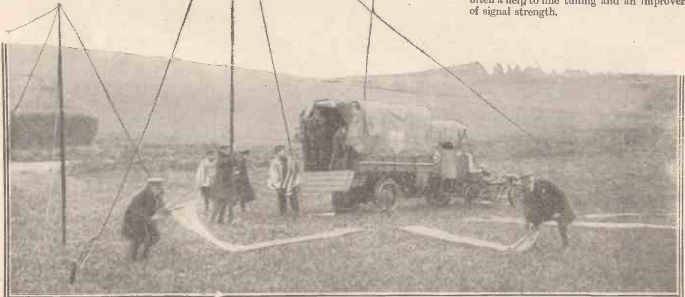
Erecting a field wireless station. The photograph shows the laying of the earth-mat—a copper gauze strip which takes the place of the more permanent "buried" earth.
