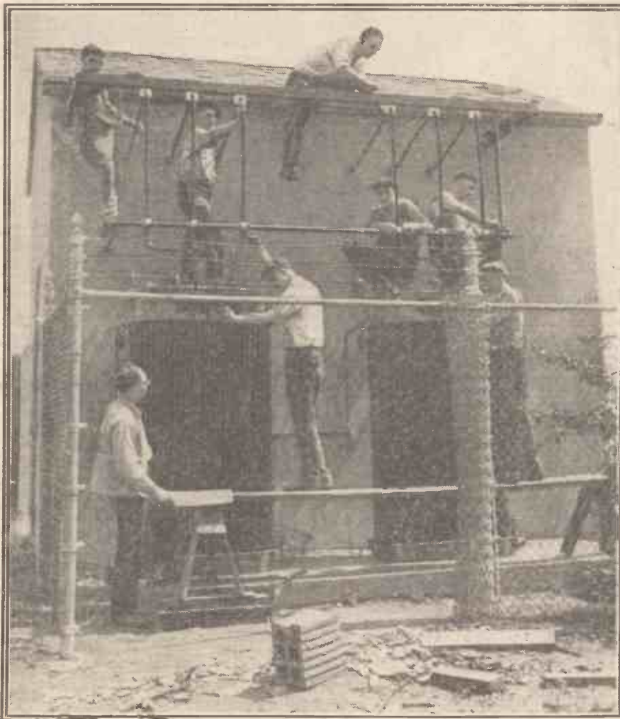
Workmen busy at work on one of the huge transformers to be employed at W J Z, an American station that is to use the immense power of 50 kw.
