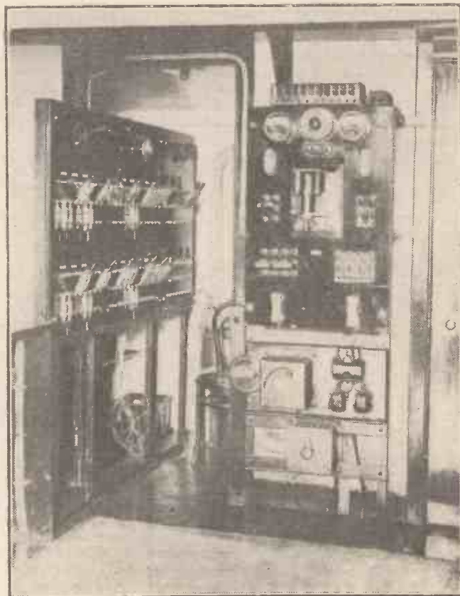
The central battery switchboard at the Glasgow broadcasting station.
