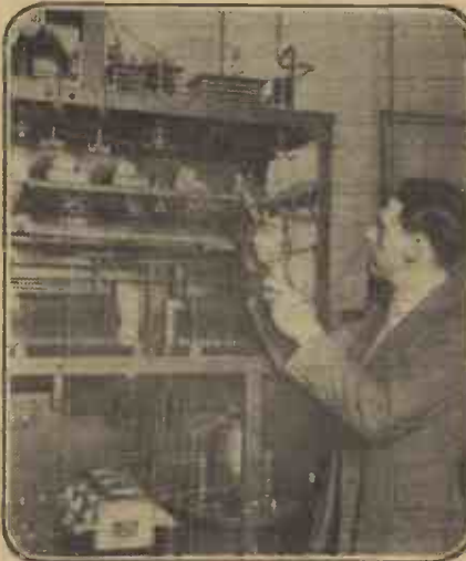
The transmitting plant at W J Z, the American broadcasting station which is to make special attempts to get over the Atlantic.
