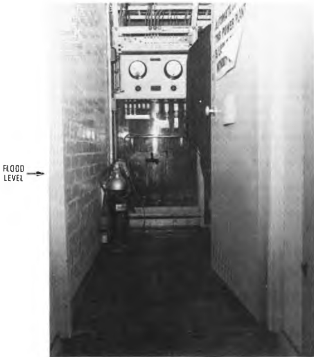
FIG. 3—The power-control rack after the flood had receded
