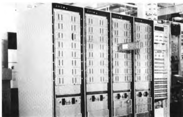
FIG. 2—The SCPC terminal equipment
