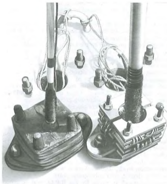
Completed shore-end anchoring clamps: exposed (right), and wrapped in preservative tape (left)
