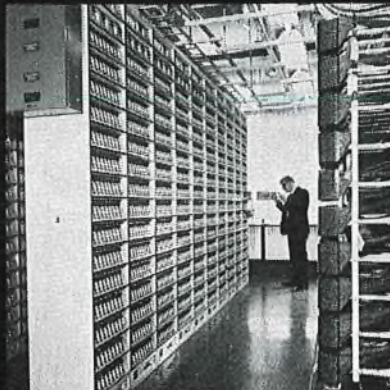
Telegraph Multiplex in London International Telex Exchange.
