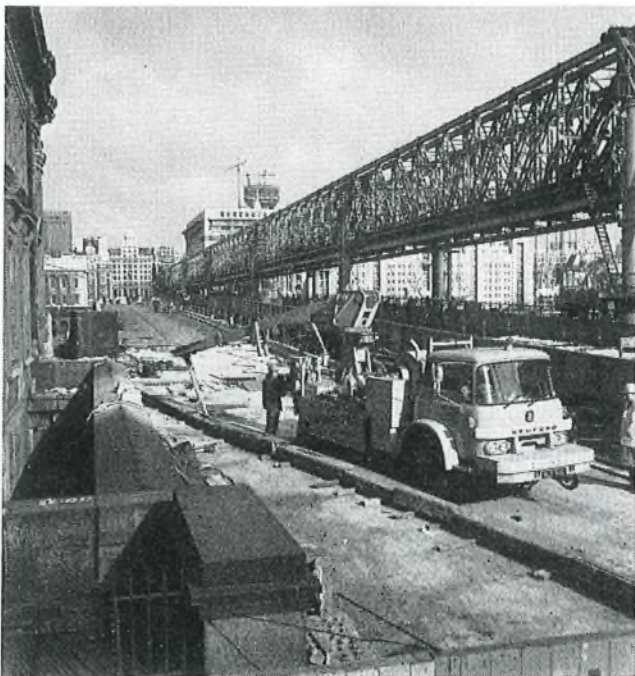
FIG. 1—Heavy cabling unit preparing to pull cables in at the south side of London Bridge
