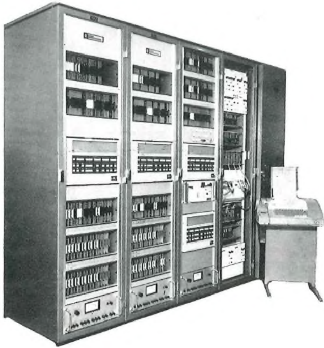
From left to right this photograph shows two translator cabinets, a common-equipment cabinet and two magnetic-drum cabinets.
