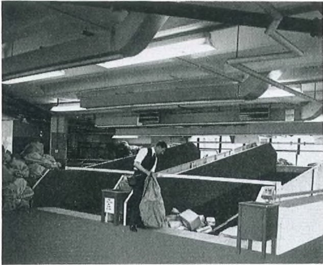
FIG. 4—Vertical riser discharge chute
