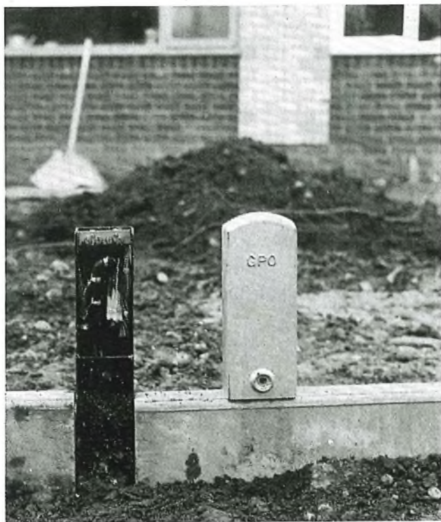
ABOVE-GROUND JOINTING POST
