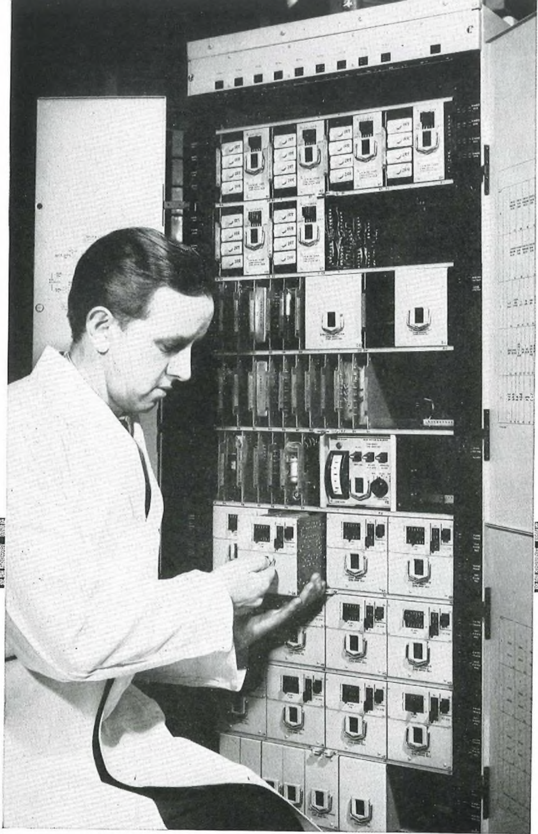
Typical Type C12G terminal rackside
