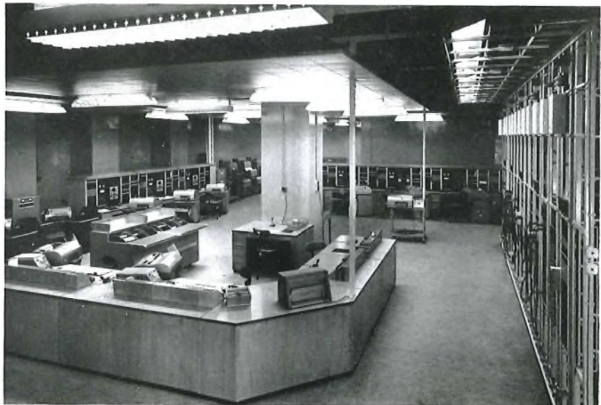
In the foreground are maintenance-control positions. FIG. 5—GENERAL VIEW OF TEST ROOM
