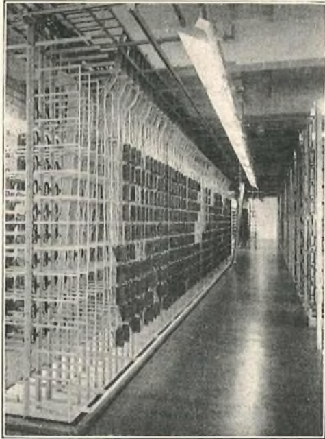
FIG. 5.—ILLUMINATION OF I.D.F. USING FIXED FLUORESCENT LIGHTING FITTINGS.
