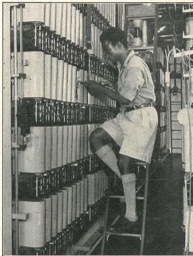
By courtesy of Nigeria Trade Journal and the Federal Information Services LAGOS AUTOMATIC EXCHANGE, EQUIPPED WITH PRE-2,000-TYPE SWITCHES. NEW EXCHANGES ARE BEING EQUIPPED WITH S.E.50 SWITCHES.
