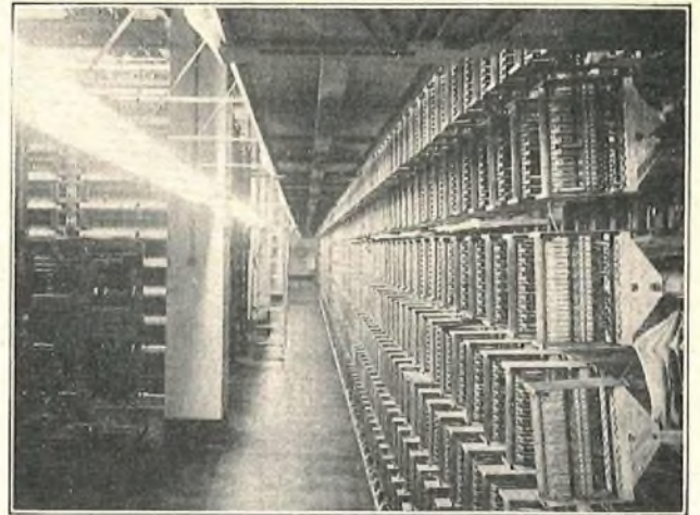
FIG. 7.—ILLUMINATION OF LOWER PART OF M.D.F. WITH MEZZANINE PLATFORM, USING FLUORESCENT LIGHTING WITH CONTINUOUS REFLECTOR.
