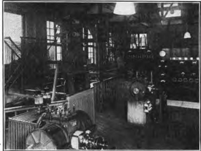
FIG. 1.—NORTHOLT RADIO STATION: POULSEN ARC TRANSMITTER, WITH VALVE TRANSMITTER IN THE BACKGROUND.
