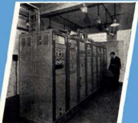
SHF repeater equipment—Manchester & Kirk o'Shotts T.V. link, 1952
