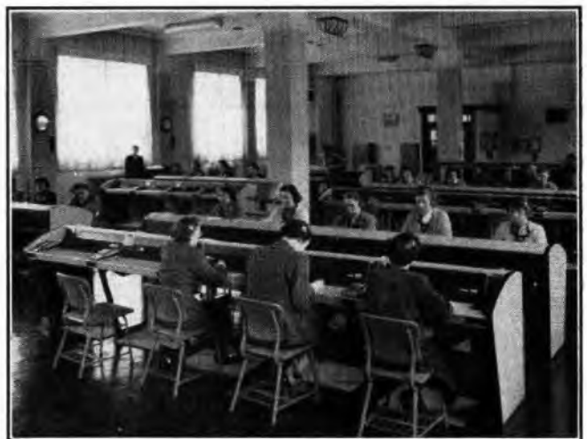
FIG. 16.—CORDLESS SWITCHBOARD AT THANET EXCHANGE.
