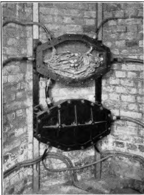
FIG. 12.—AN EARLY CABLE DISTRIBUTION HEAD.
