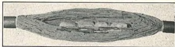
FIG. 5.—"UNICOILS" AND BUILDING-OUT CAPACITORS INSERTED IN CABLE JOINT.
