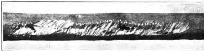
DAMAGE CAUSED BY SQUIRREL TO 15-PAIR L.C. CABLE.
