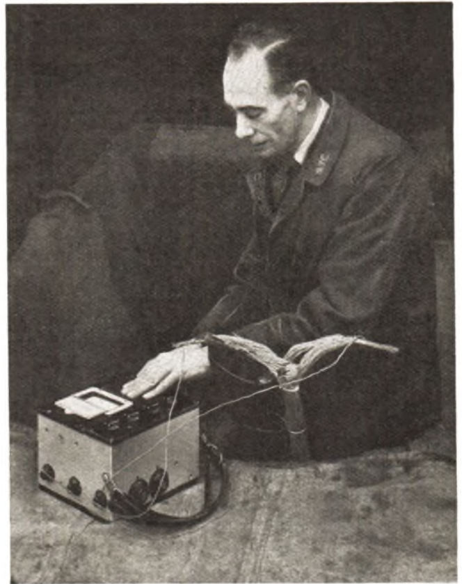
A Bridge-Megger Tester, Series 2, in use by the Post Office Engineering Department. The engineer is shown testing the insulation of 300 pair 6½ lb. P.C.U.T. cable at a pavement box.
