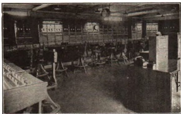
THE SWITCHROOM, ROYAL SHOW EXCHANGE, OXFORD.
