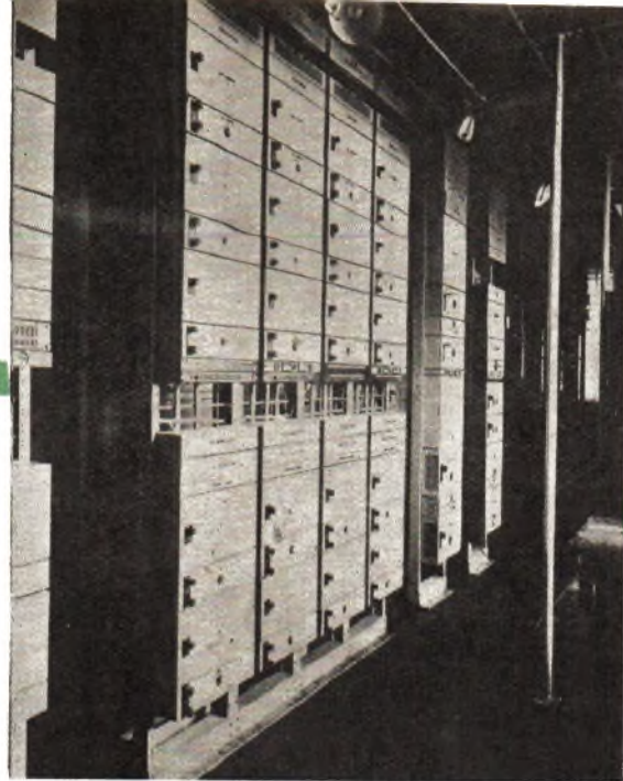
Coaxial system bays at Kidderminster.
