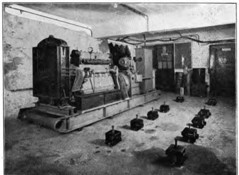
FIG. 7.—DAVEY PAXMAN 65-KVA SET WITH ANTI-VIBRATORS AT CLERKENWELL EXCHANGE.
