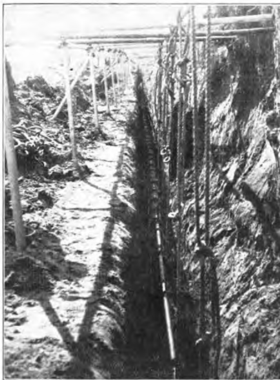
GENERAL VIEW OF METHOD OF SUPPORTING 3-WAY DUCT DURING LOWERING AT SINDERBY.
