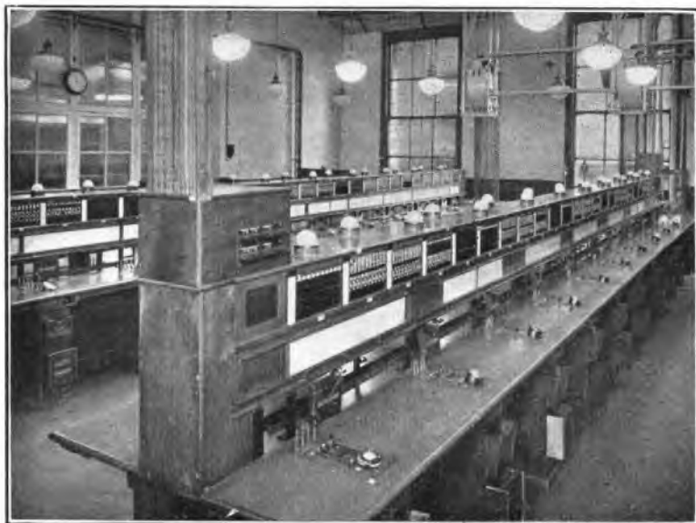
FIG. 1.—THE PHONOGRAM SWITCHROOM AT NEWCASTLE, EQUIPPED WITH DOUBLE-TIER ANCILLARY SWITCHBOARDS.
