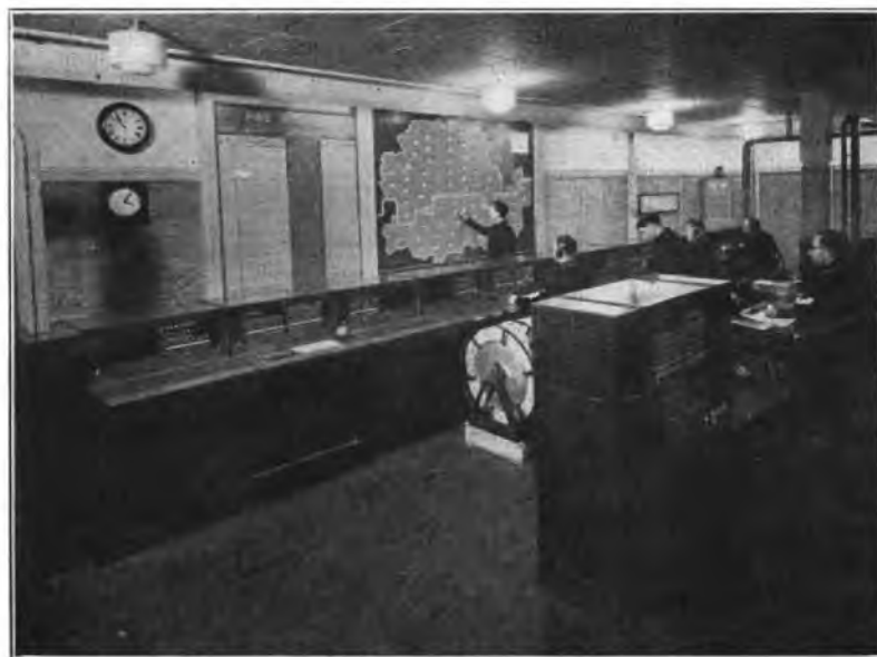
FIG. 1.—GENERAL VIEW OF SWITCHROOM.
