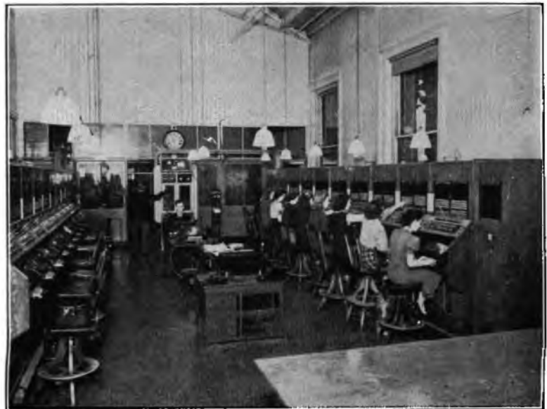
FIG. 6.—TELEPRINTER SWITCHBOARDS AT MANCHESTER.
