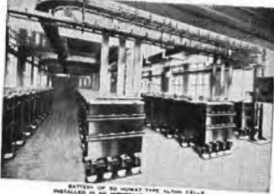
BATTERY OF 50 HENRY TYPE ALTON CELLS INSTALLED IN AN IMPORTANT LONDON ESTABLISHMENT
