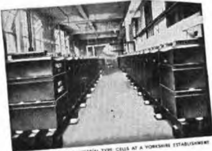
TWO ALTON BATTERIES OF JUV27/31 TYPE CELLS AT A YORKSHIRE ESTABLISHMENT
