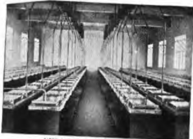
ALTON BATTERY OF 254 SWH TYPE CELLS AT A CORPORATION ELECTRICITY WORKS
