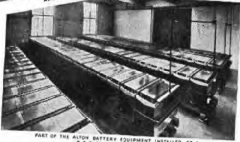
PART OF THE ALTON BATTERY EQUIPMENT INSTALLED AT A B.B.C. TRANSMITTING STATION
