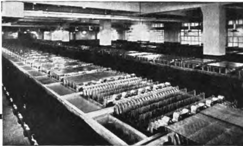
Illustration shows an installation of Alton Batteries of Merit at an important London Telephone Exchange.
