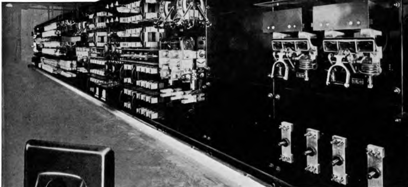
We are indebted to Messrs. William Lucy & Co. Ltd., of Oxford, the Electrical Manufacturers, and Messrs. Rankin, Phipps & Co. Ltd., the Electrical Contractors, for permission to publish this photograph.
