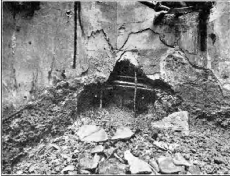
FIG. 3.—FURTHER EFFECTS OF SULPHATE CORROSION.
