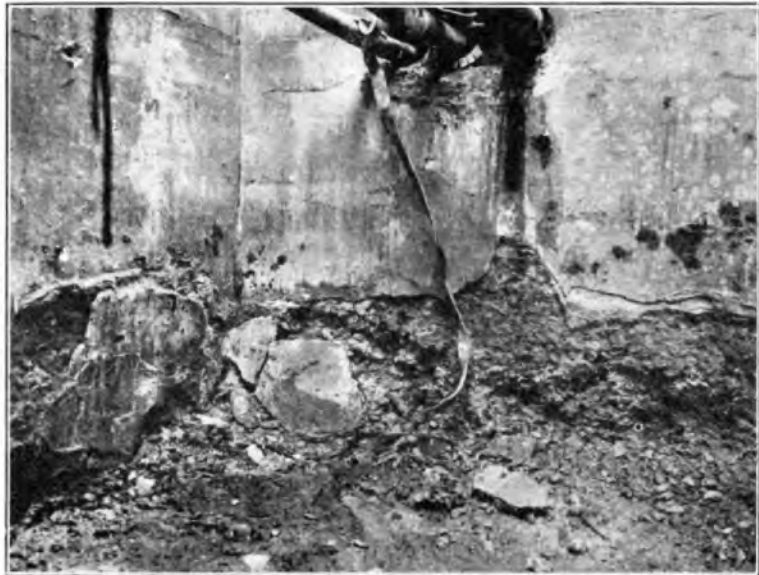
FIG. 2.—EFFECT OF SULPHATE CORROSION.
