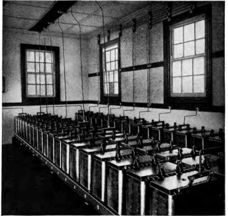
Illustration shows battery of 120 " BRPG 19 " type ALTON cells installed at Slangkop Wireless Station, which is the main " Coast-to-Ship " radiogram station for the Union of South Africa.
